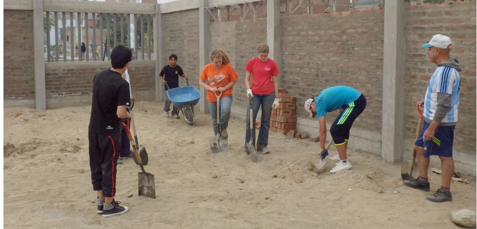
Greyfriars students Megan Snyder and Celina McGowan work alongside church members in Peru, constructing an education building
